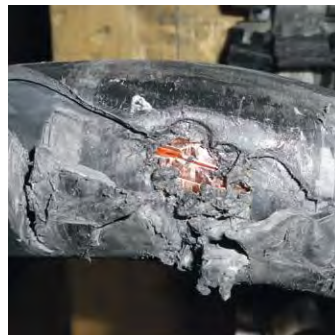
Major cable damage caused by thread contact
