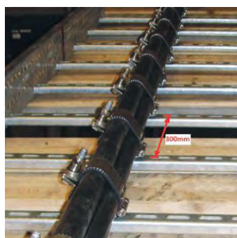
Before short circuit test
